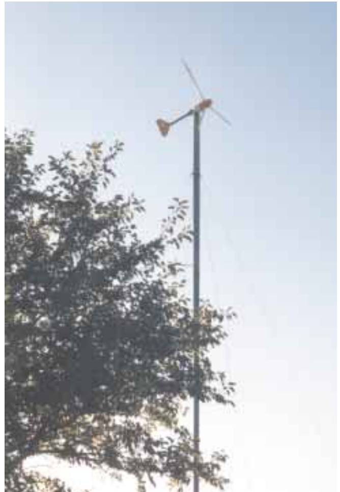
The 10 KW Bergey Excel powers the town water supply.
