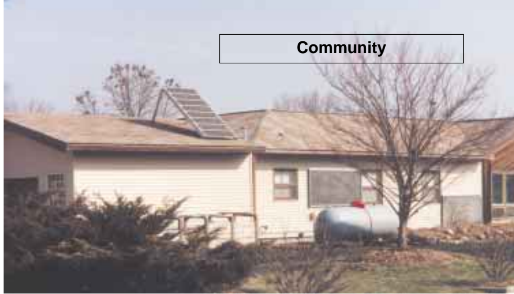
Russ Hardtke has eight Arco Solar 16-2000 PVs and solar hot air collectors.
