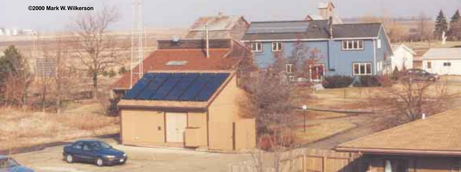
The Stelle community phone system (foreground) utilizes 2,900 watts of PV.
